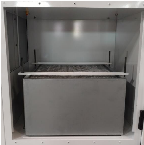
Figure 6: HEPA filter shown installed
